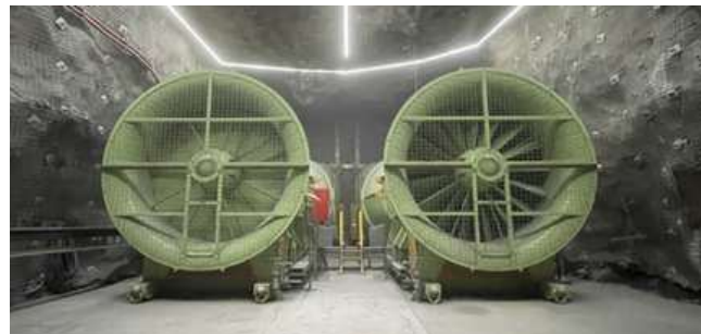
New underground ventilation fans
